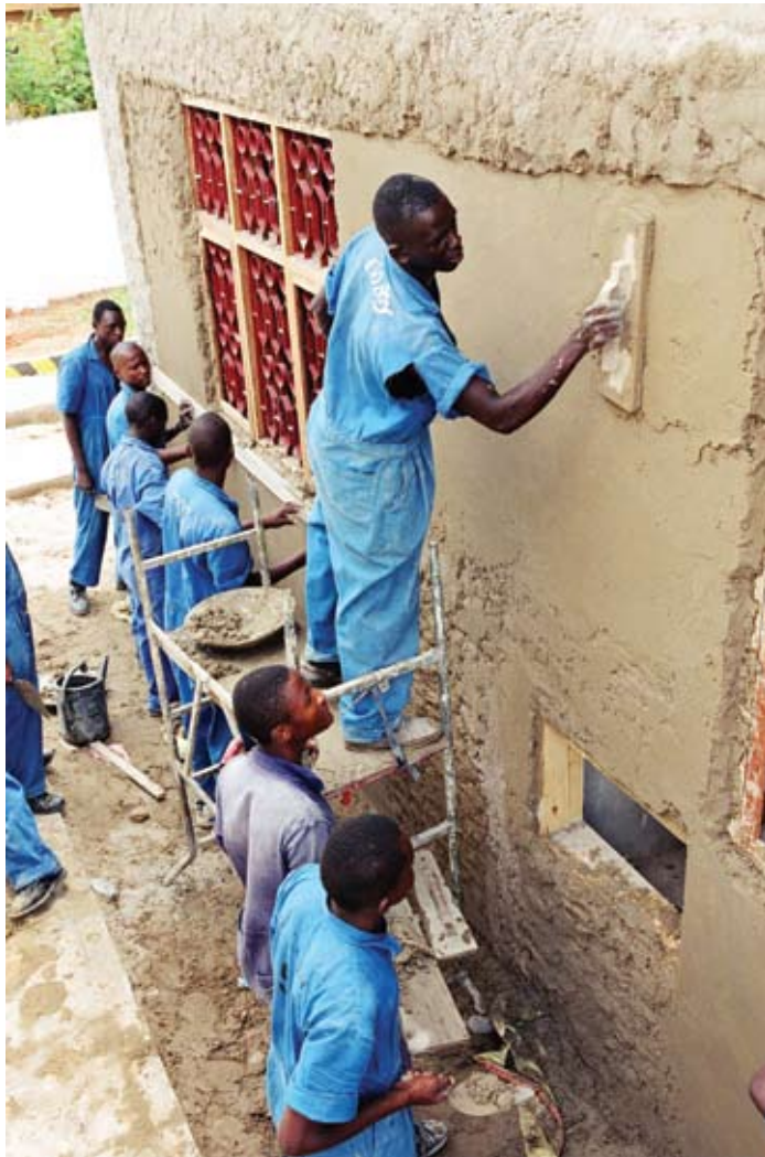
Training is one element in promoting decent work in the construction industry: masonry workshop of the Dar-es-Salaam Regional Vocational Training and Services Center, October 2003. Photo: ©ILO/Crozet
