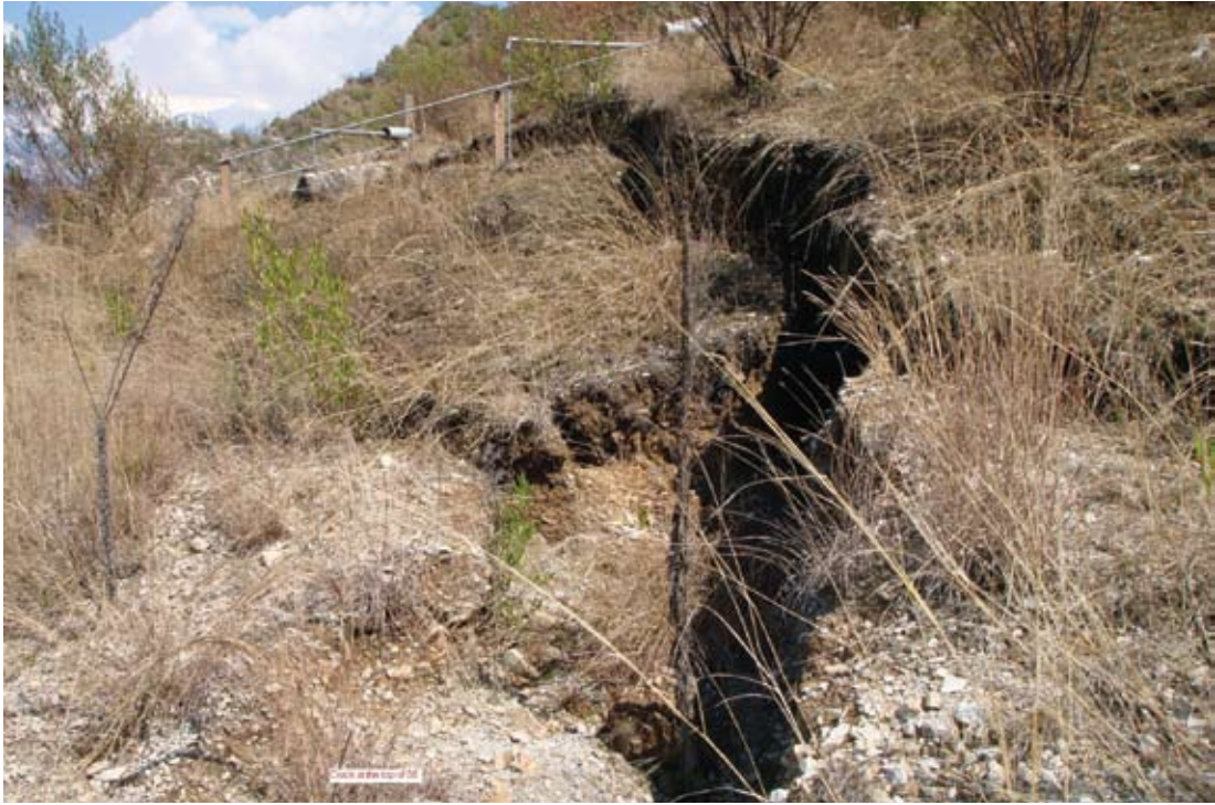
Motion detectors donated by a U.S. University for monitoring crack activity on hillsides above Muzaffarabad, Kashmir, Pakistan. Photo: Abdur Rauf Qureshi, IUCN Pakistan, 2007.
